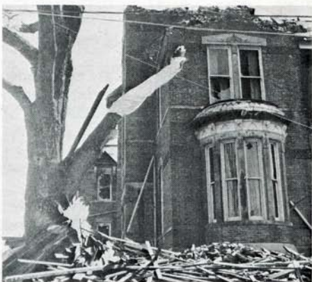
Masonic Temple after Tornado, front view.
