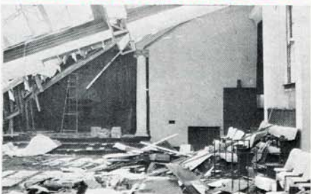
Lodge Room after Tornado, south view.
